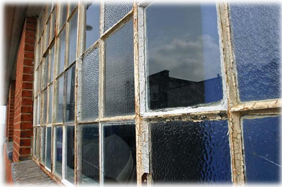
Fig. 3 Metal window demonstrating lack of maintenance
