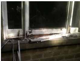
Decayed timber frame and cill
